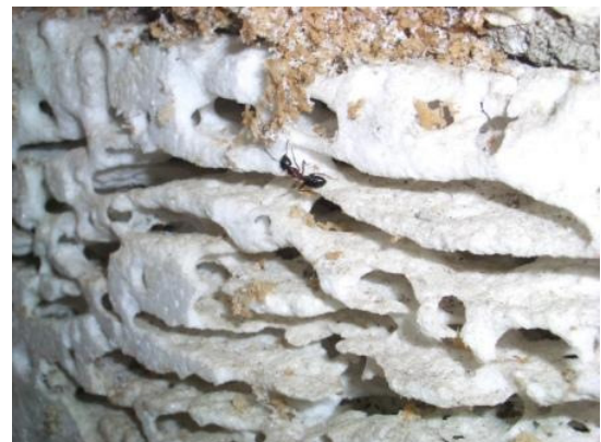
Picture 2: Damage in expanded polystyrene caused by Carpenter ants ( Camponotus ligniperda )
